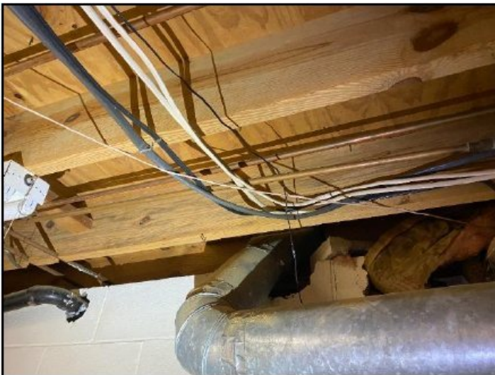
39. Too close to/touching duct, pipe, vent or...
