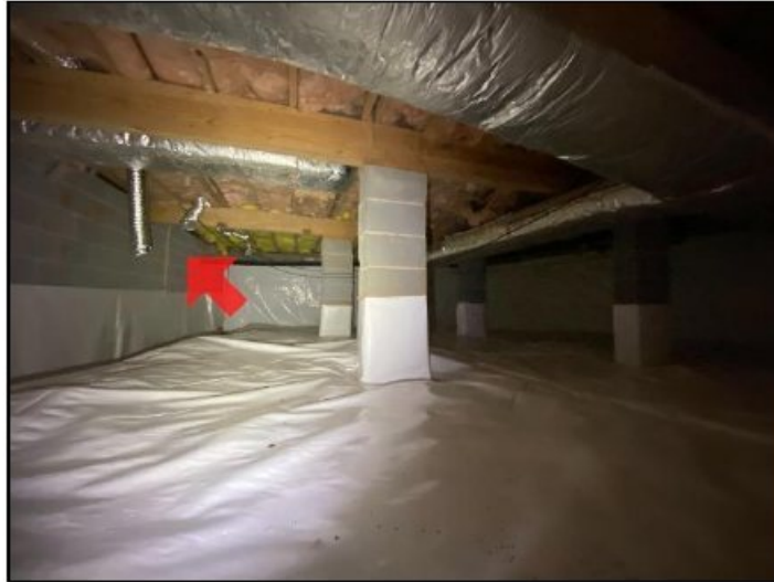
73. Dryer vent disconnected
