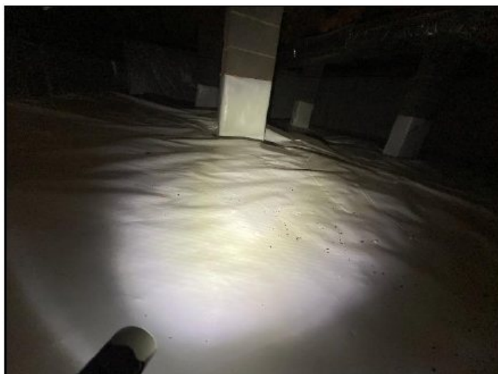
53. Animal/pest droppings in crawlspace
