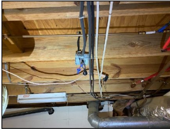
44. Cover loose or missing
