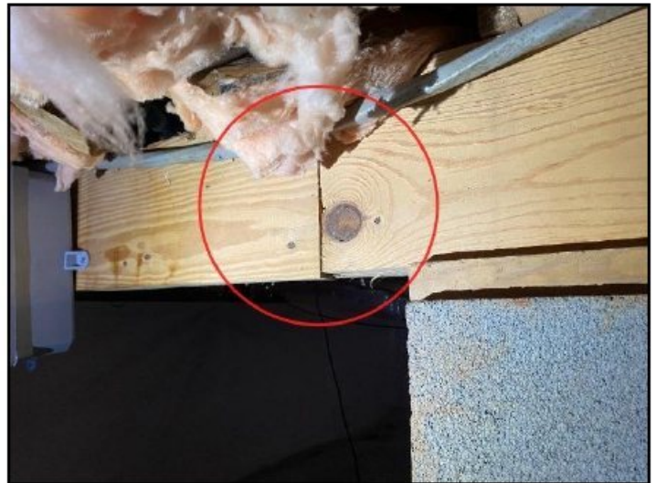
25. Poor connections in built-up beams
