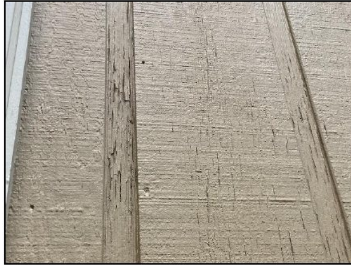
7. Paint or stain - needed
