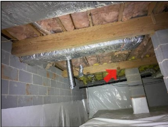
24. Poor connections in built-up beams
