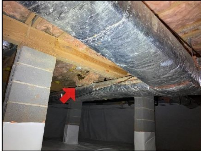
52. Loose, sagging or voids
