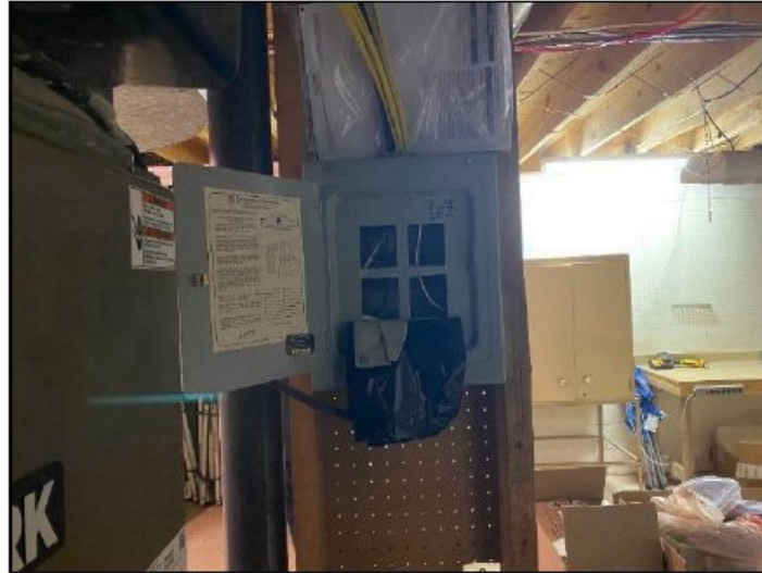
30. Obsolete service box
