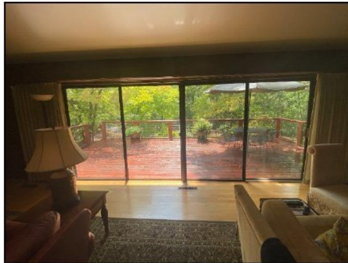
72. Safety glass not installed
