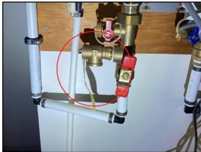
63. Discharge tube missing
